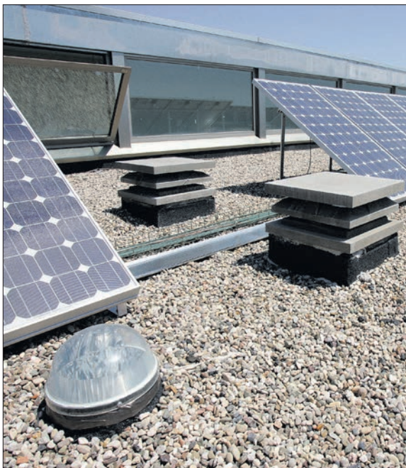
Centre Esplai. Plaques i pous solars. FOTO: FUNDESPLAI
